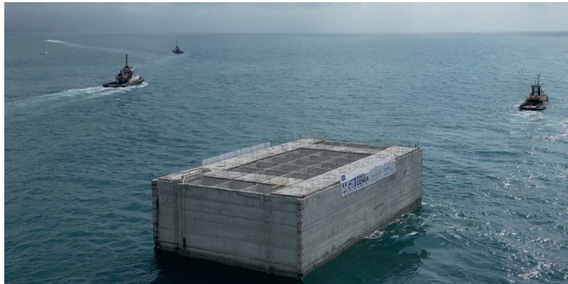
All caissons are fabricated at sea – on a barge or floating dock – at the port of Vado Ligure, 37km from Genoa (top picture). Then they are transported by boat to their assigned position (Credit: Port of Genoa)
